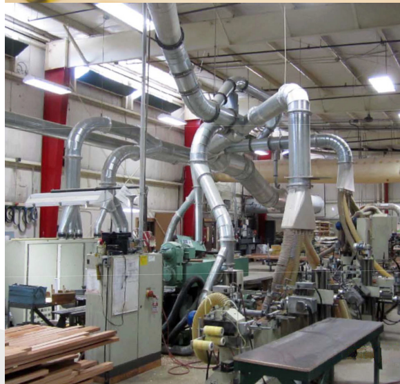
Above: Woodworking facility before installation of Nordfab ducting.
