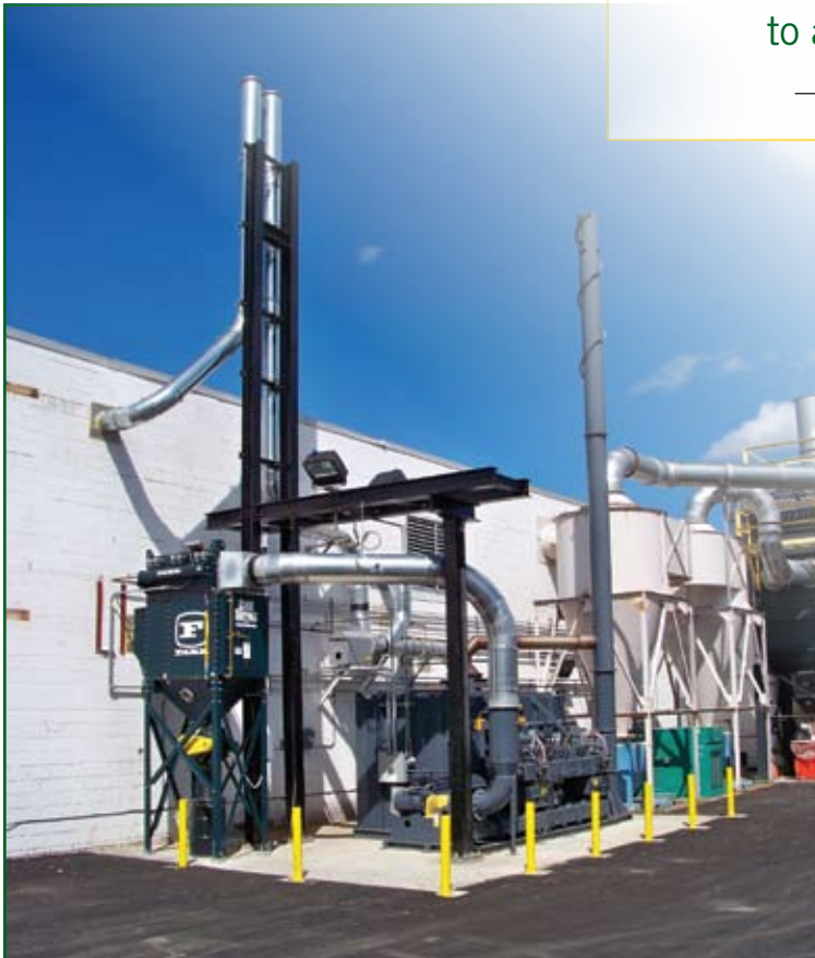
Gold Series model GS6 being used as an in-line pre-filter for a thermal oxidizer.
